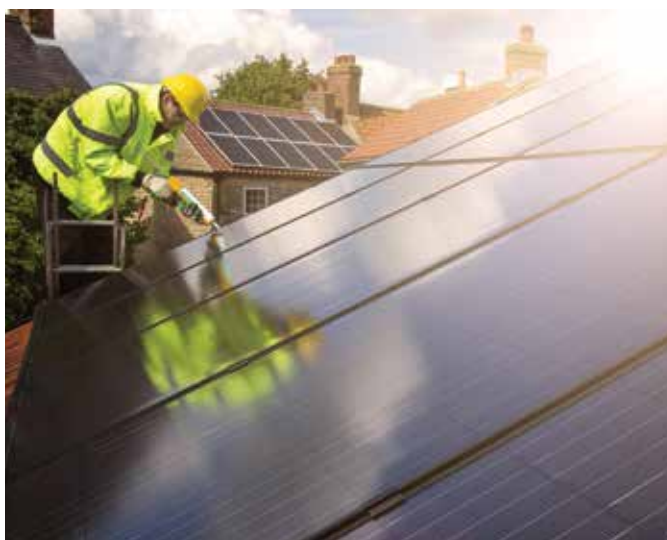
Installation of solar panels is contributing to a reduction in our Co 2 emissions
